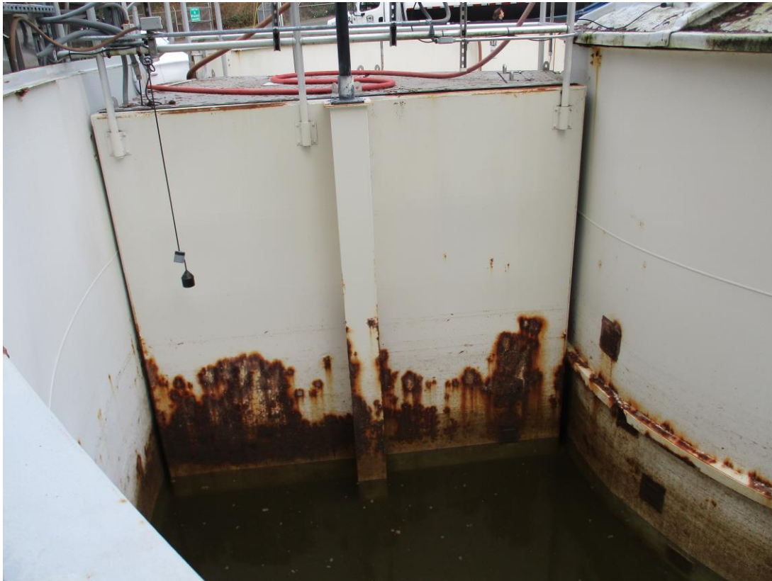
Photo 2 – Corrosion at the EQ Basin
