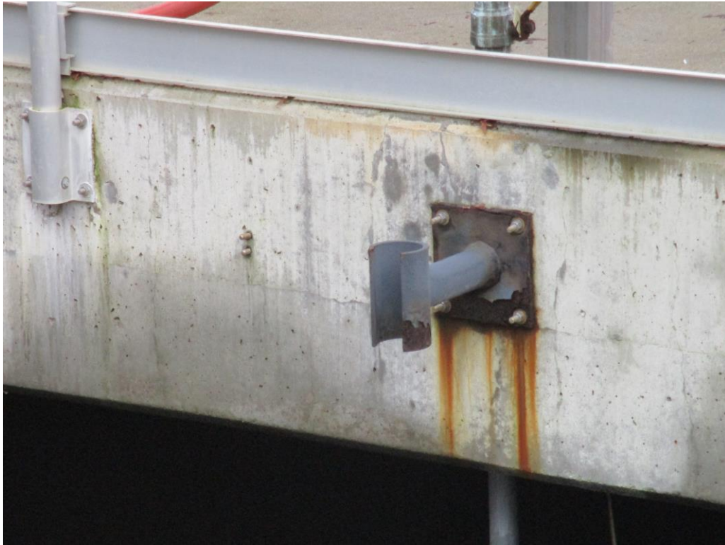
Photo 5 – Corrosion of Metal Plate at SBR Basins
