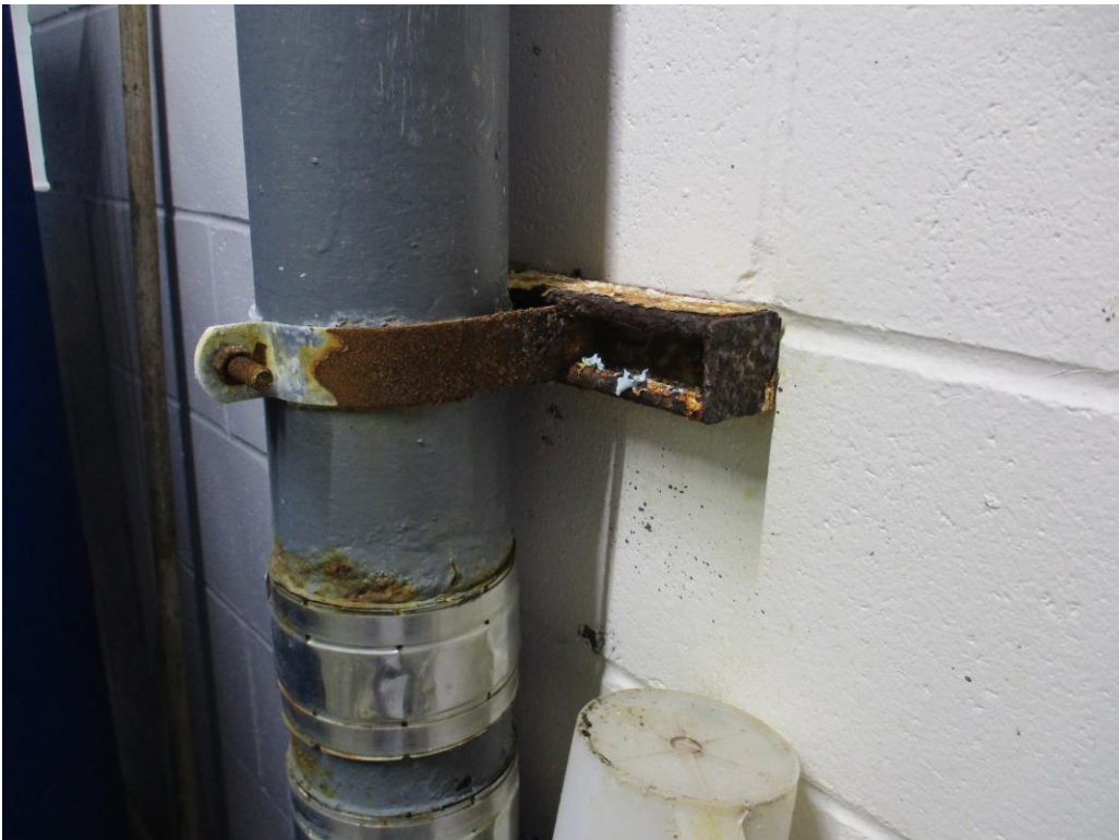
Photo 8 – Corrosion of Metal Component in Process Building (Upper Floor)
