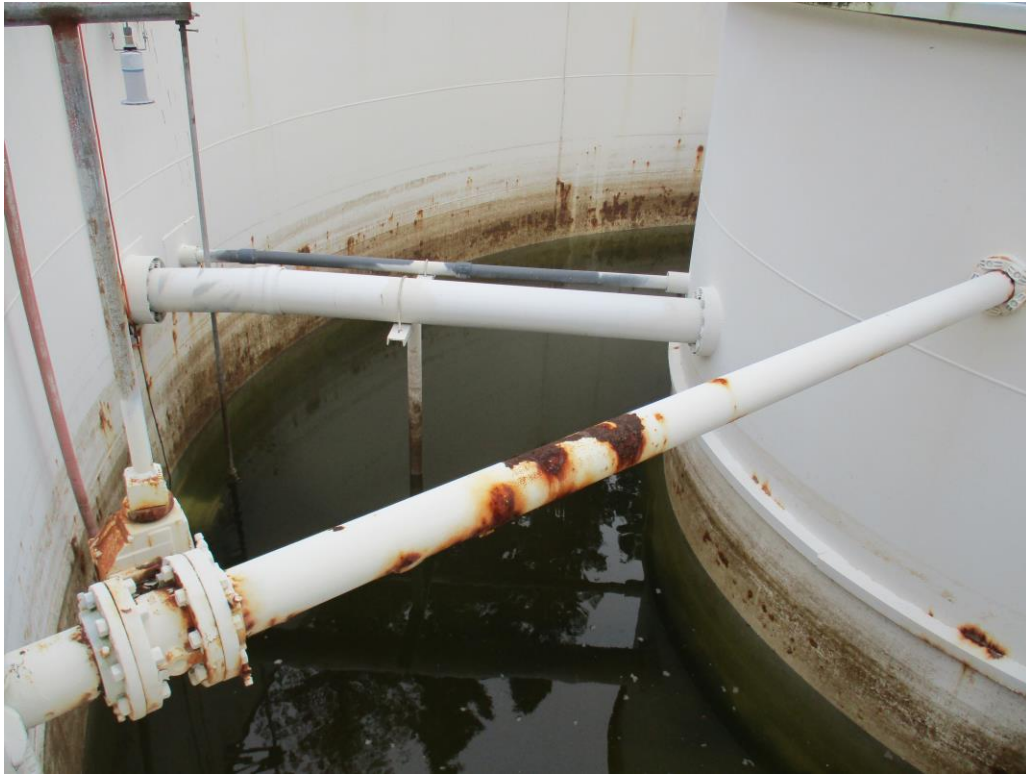
Photo 3 – Corrosion of Piping at the EQ Basin
