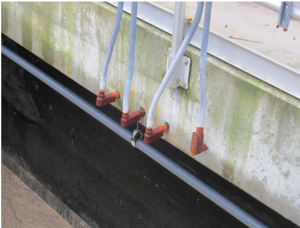
Photo 6 – Corrosion of Metals at SBR Basins
