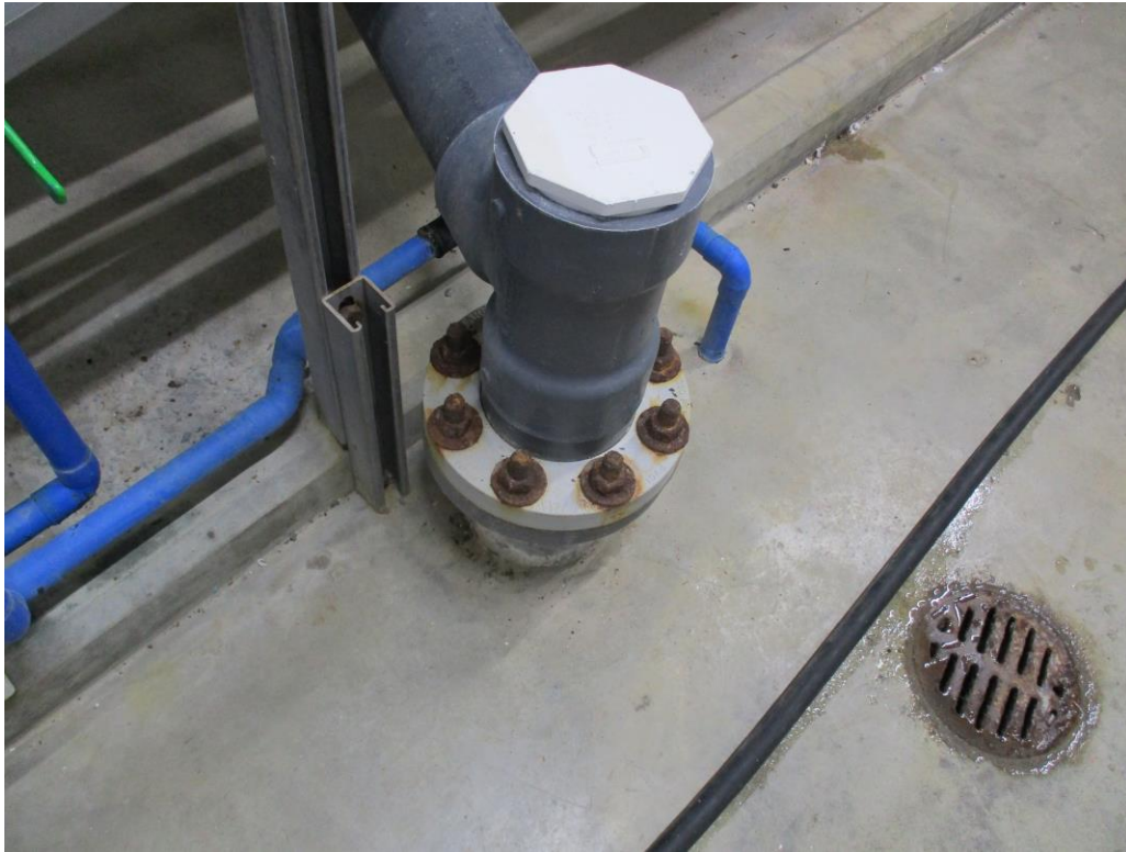
Photo 9 – Bolt Corrosion at Process Building (Upper Floor)
