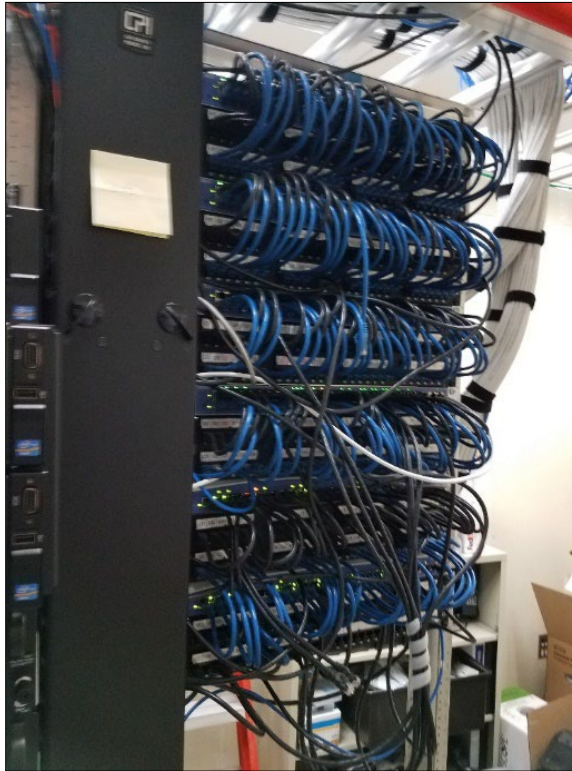
Photo 1. Example of Cable Management inside SRV-1
