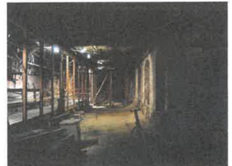
The concrete floor of the former meat market was originally at the level of the wooden platform on the left but sank over time because of decomposing sawdust fill.
