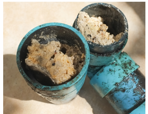
A sewer pipe clogged with F.O.G.
