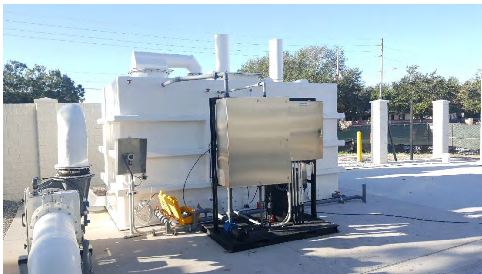
Figure 8-9 | OC-3 Engineered Biofilter
