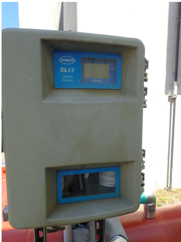
Figure 3-16. CKTP reclaimed-water filtration system chlorine residual analyzer powered down
