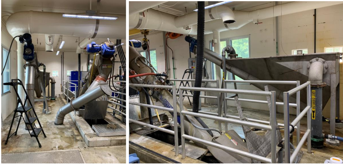
Figure 5 – STP Headworks Room
