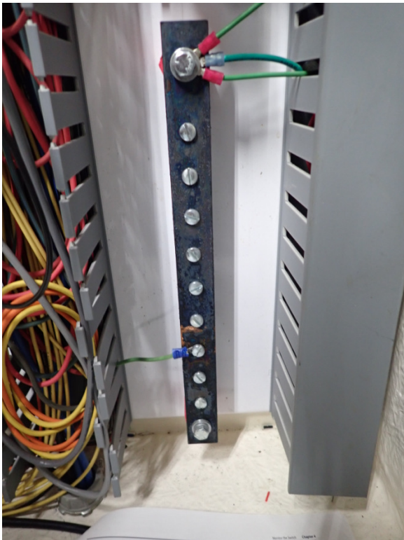
Figure 3-7. H_2S corrosion on digester control building control panel (PNL 6000) copper ground bar
