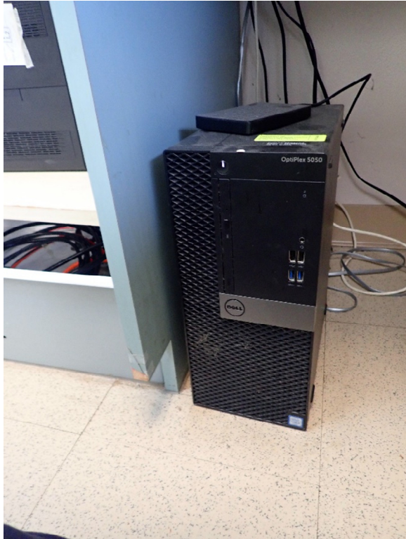
Figure 2-26. KWWTP SCADA PC with connected external hard drive
