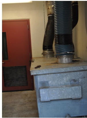
Grit and Screenings Bin
