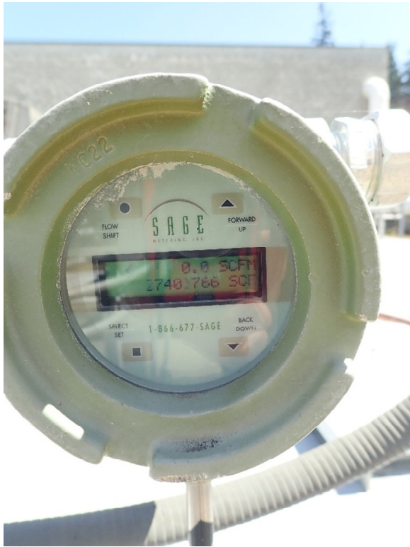
Figure 3-18. CKTP aerated grit tank 1 stage 2 flowmeter reading zero flow
