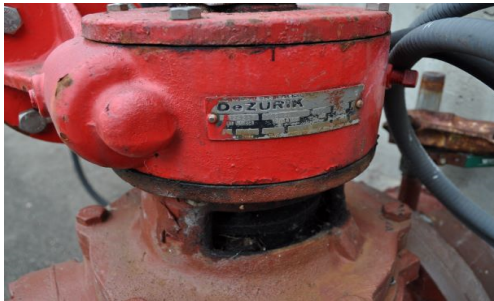
FV-42-1 AB 1 effluent piping control valve
