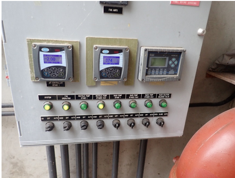
Figure 3-19. MWWTP odor control system control panel instrumentation
