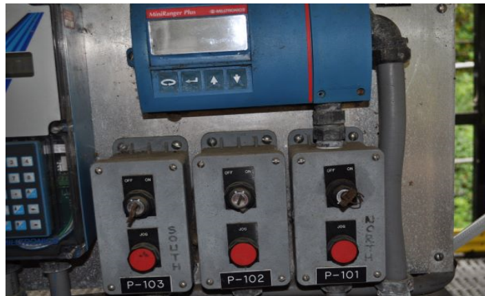
Influent Pump Station Controls
