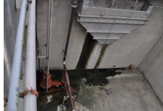
AB Jet Aeration Pump and Effluent Weir
