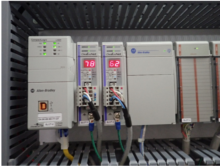
Figure 3-5. DeviceNet scanners in PNL 2939 PLC rack
