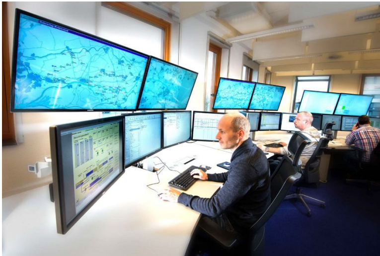
Figure 5-1. Example four-monitor operator workstation configuration with large-format displays
