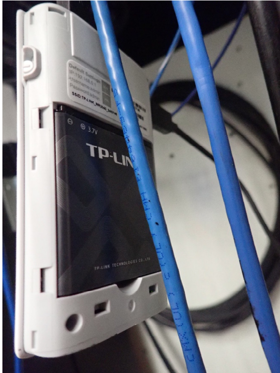
Figure 2-16. TP-Link MR3040 cellular router connected to OT network unmanaged switch
