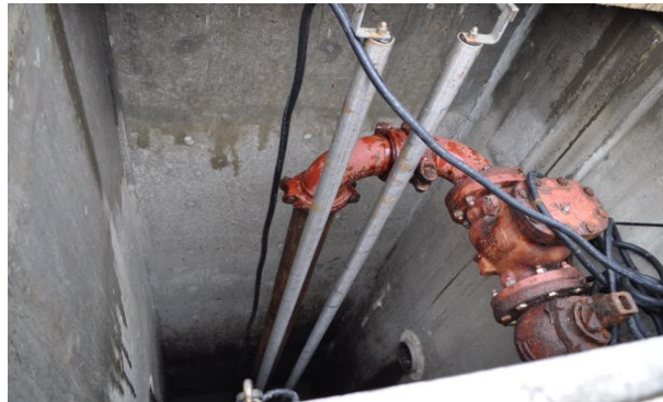
Scum wetwell interior and scum pump P-405
