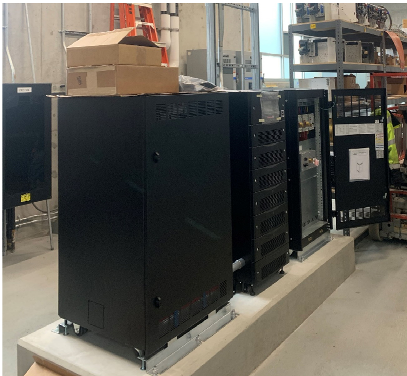
Figure 5-10. Example three-phase UPS system recently installed at a local wastewater utility
