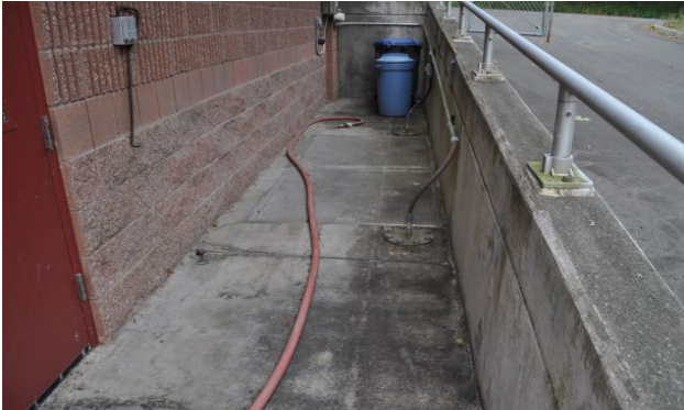
WAS tank exterior
