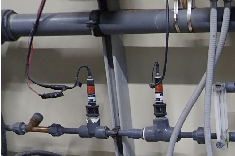
Figure 3-23. SWWTP odor control system analytical probe with splice in manufacturer cable
