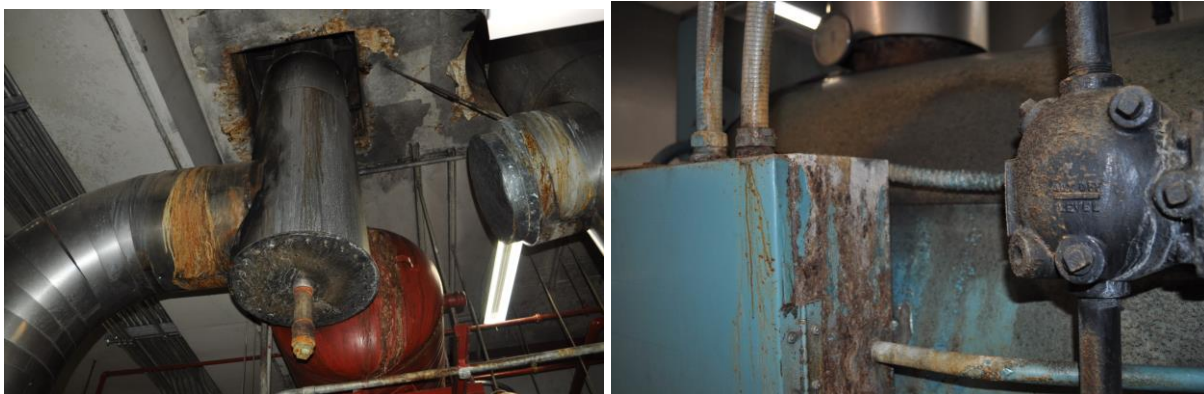
Figure 3 – Rusty Boiler Components due to the Leaking Roof Penetrations
