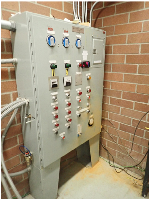
Figure 3-31. PS-34 control panel
