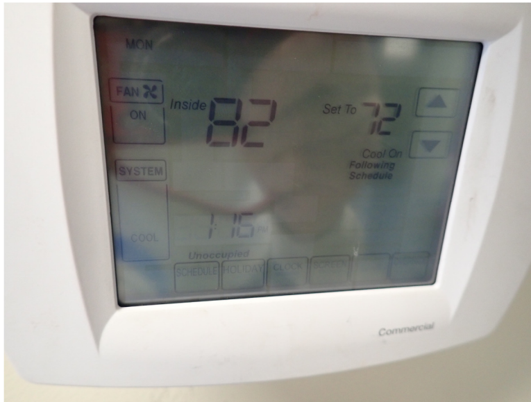
Figure 3-8. Headworks building electrical room thermostat
