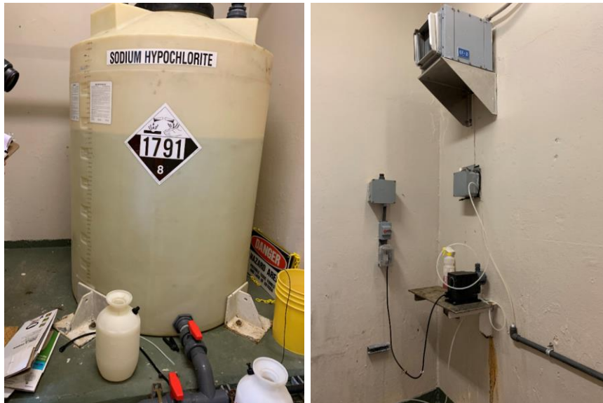
Figure 4 – MTP Sodium Hypochlorite Storage Room
