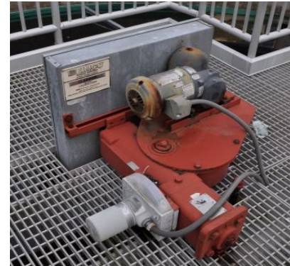
M-402 Secondary Clarifier Drive
