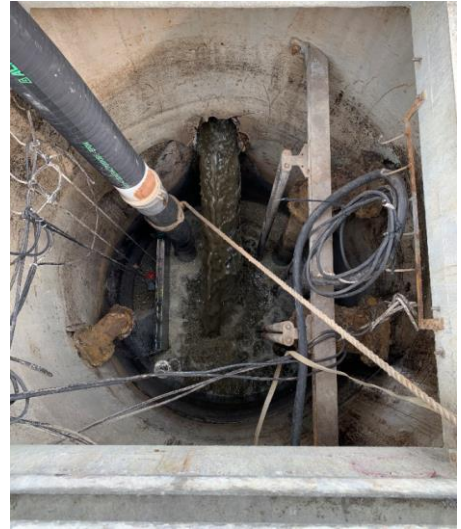
Figure 2 – CKTP In-Plant Pump Station
