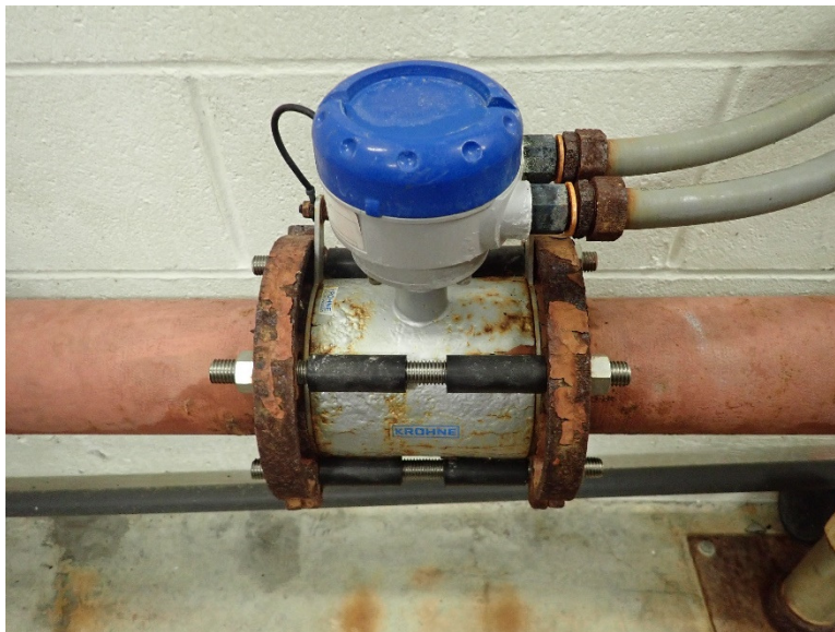
Figure 3-20. Corroded magmeter on sludge line to MWWTP gravity belt thickener
