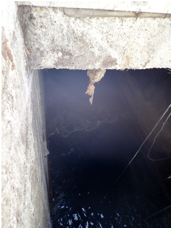
Figure 3-30. PS-24 wet well ultrasonic level transducer coated with grime and dried scum
