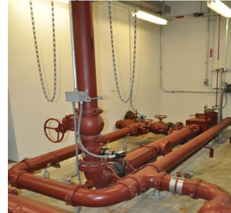
P-611 Sludge Pump
