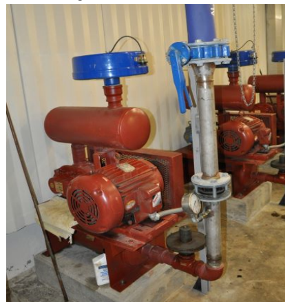
B-601-603 Sludge Tank Blowers
