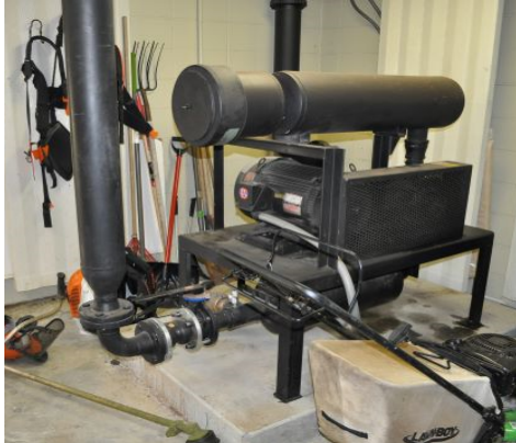
Aeration Basin Blower
