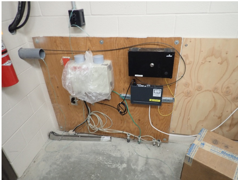
Figure 2-17. KWWTP operations building electrical room communications backboard
