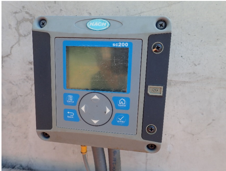
Figure 3-17. CKTP reclaimed-water filtration system turbidity analyzer powered down
