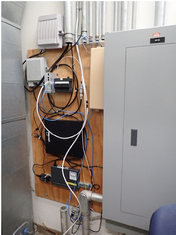
Figure 2-18. MWWTP operations building electrical room communications backboard
