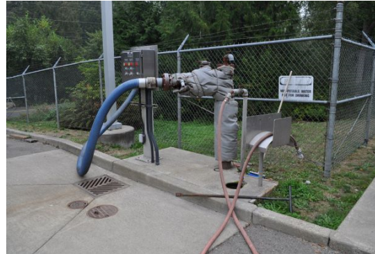
Truck Filling Station
