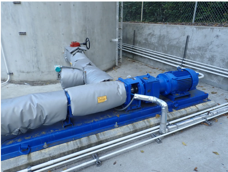
Figure 3-25. SWWTP thickened sludge tank level transmitter on truck loadout pump suction piping
