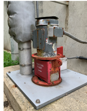
P-175 Odor Control Blowdown Pump
