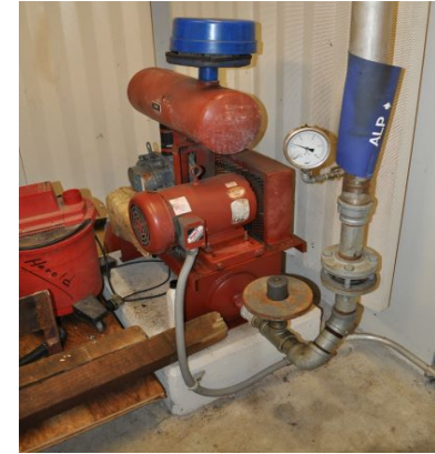
B-211 Channel Aeration Blower
