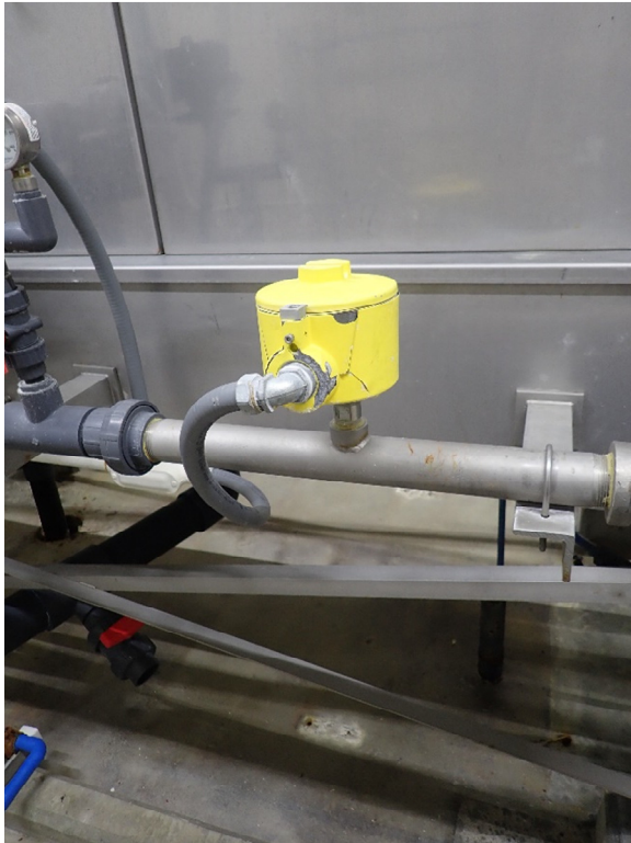
Figure 3-28. Damaged flow switch on SWWTP RDT spray water supply line
