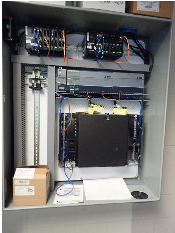
Figure 2-3. Modular access switches in PNL 8580A
