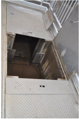
ML Splitter Box to Secondary Clarifiers
