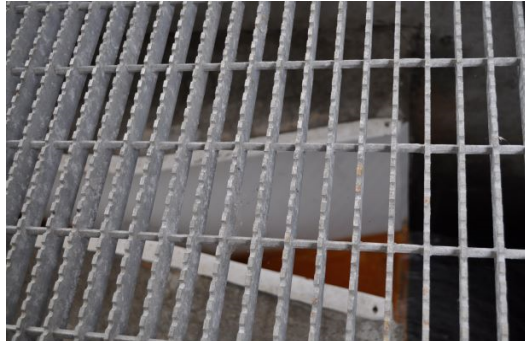
M-505 Effluent Parshall Flume
