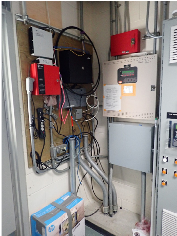
Figure 2-19. SWWTP process building electrical room communications backboard
