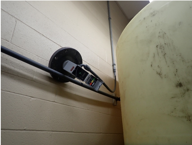
Figure 3-32. Failed ultrasonic level probe disconnected from PS-71 BIOXIDE storage tank
