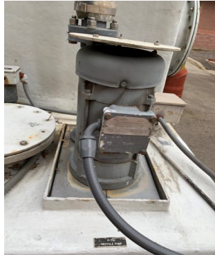
P-701 Recirculation Pump
