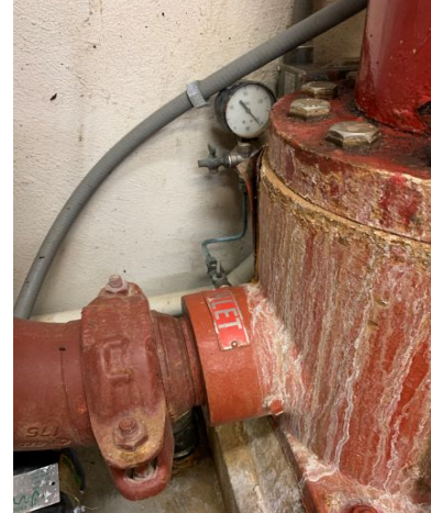
W3 Automatic Strainer corrosion
