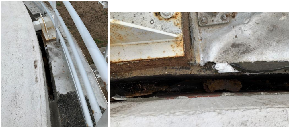
Figure 1 – CKTP Digester 2 Seal Failure
