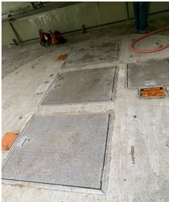
Influent Pump Station
