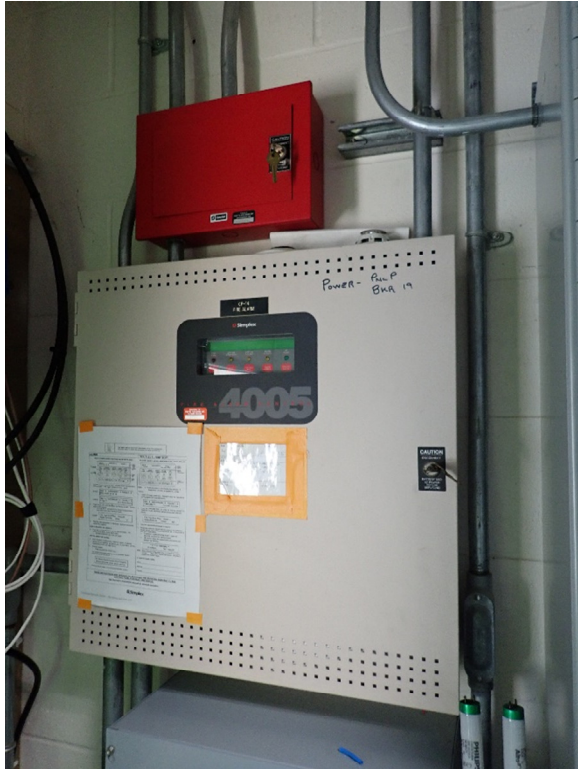
Figure 3-27. Failed fire alarm system panel at SWWTP process building
