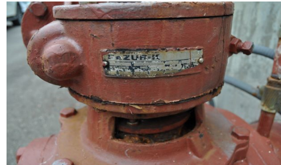
FV-42-2 AB 2 effluent piping control valve
