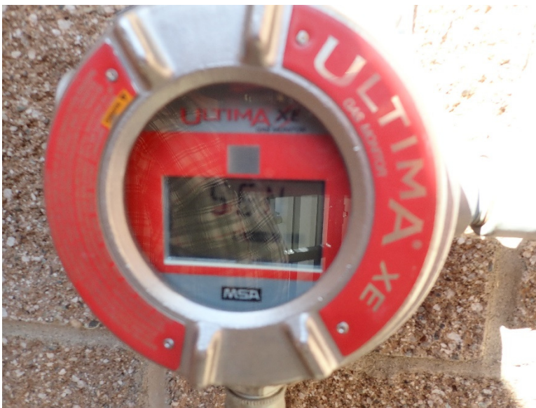
Figure 3-33. PS-71 wet well LEL monitor in alarm
