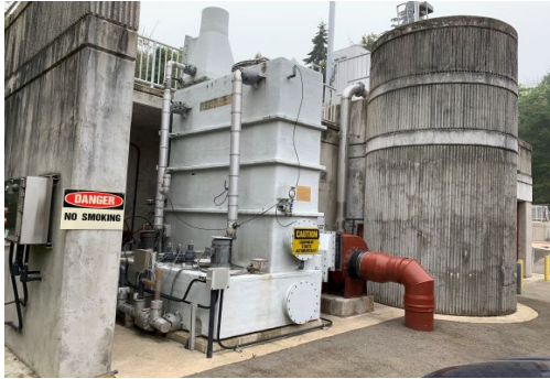
Odor Control System
