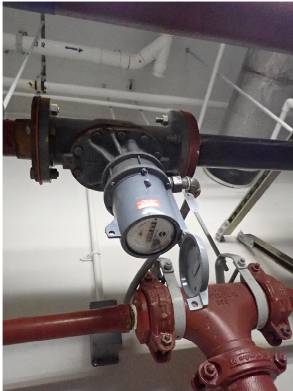
Figure 3-22. MWWTP W3 pump flow transmitter and totalizer
