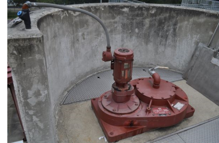
M-210 Grit Chamber
