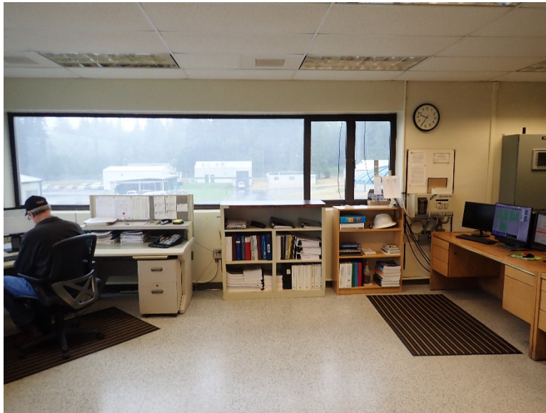
Figure 3-10. CKTP SPB control room
