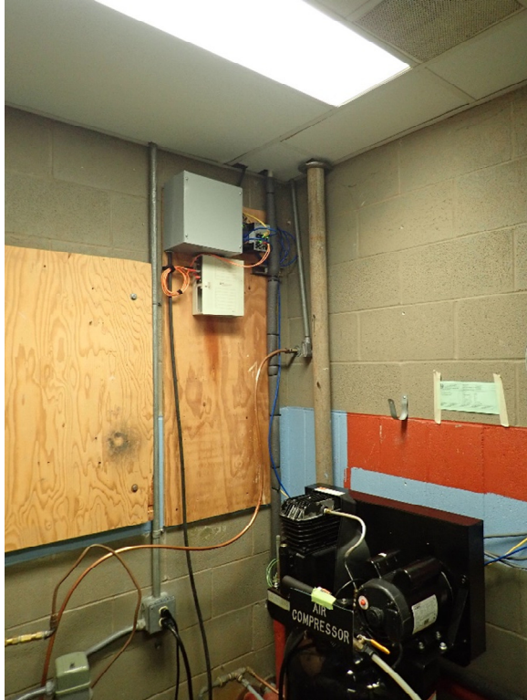
Figure 2-24. Exposed plumbing next to network components in CKTP administration and lab building electrical room
