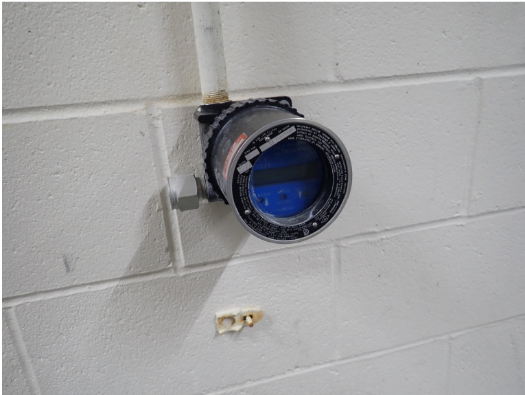
Figure 3-24. Non-functional LEL gas monitor in the SWWTP process building upper-floor process room
