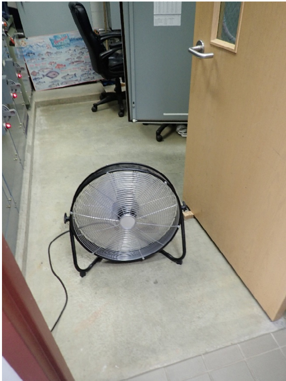
Figure 3-9. Temporary ventilation measure for MWWTP electrical room
