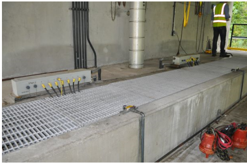
UV Power Distribution Center
