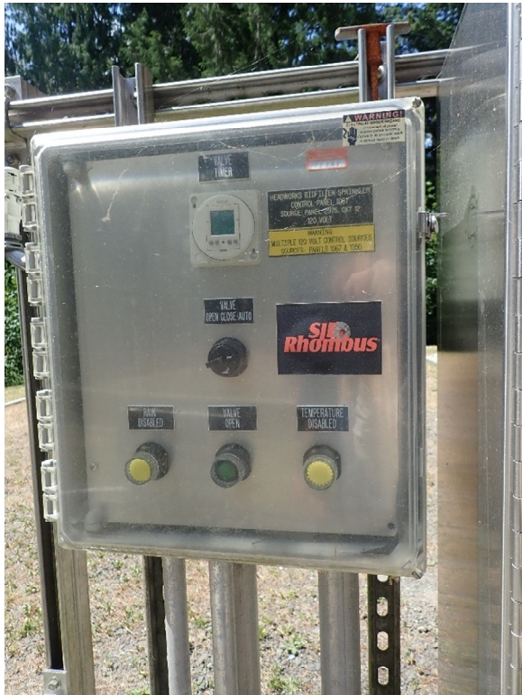
Figure 3-14. Out-of-service headworks odor control biofilter sprinkler control panel
