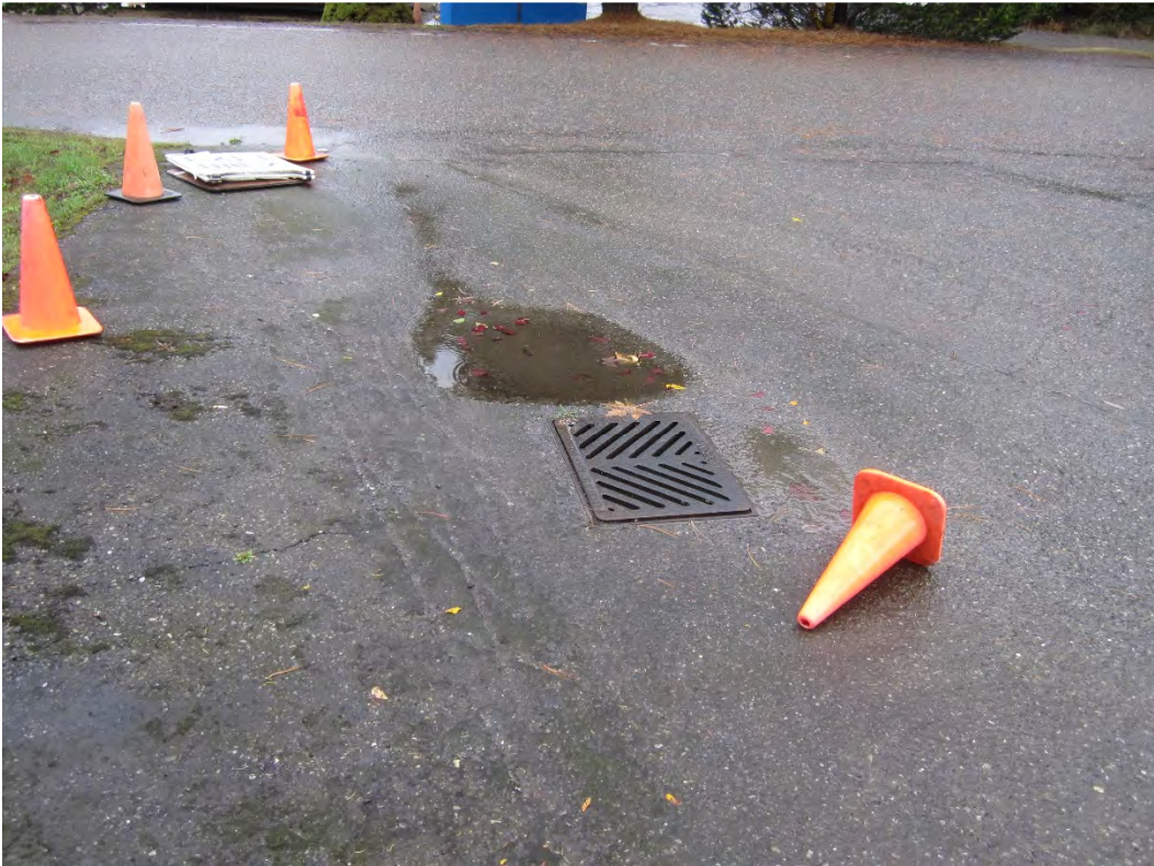
Figure 4: Ponding West of Refuse Shed C
