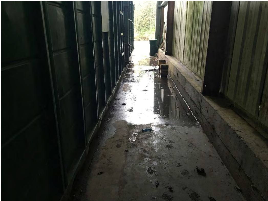
Figure 12: Pooling within Roll-Off Container Guide Rails
