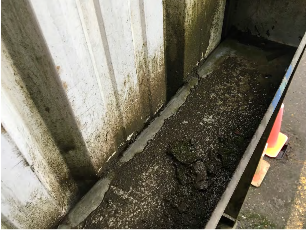
Figure 7: Wall Purlin Dirt and Moss
