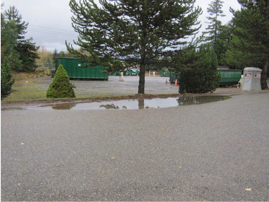
Figure 5: Ponding along the Entrance Queue Roadway
