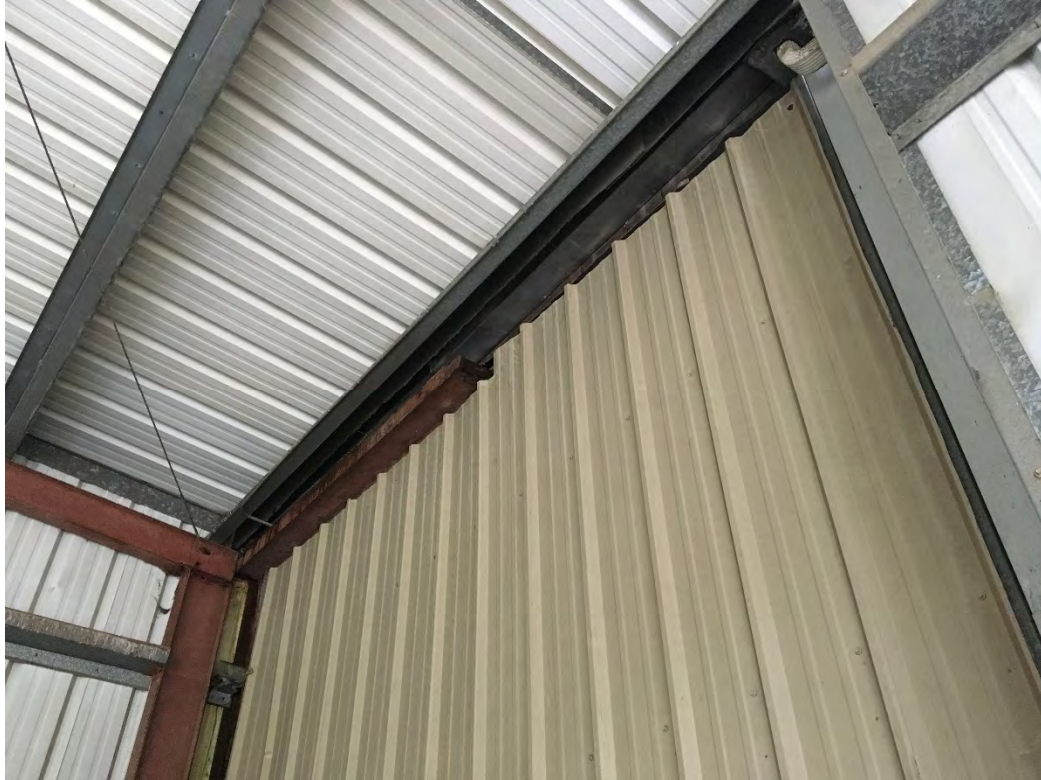
Figure 3: Leakage in the Valley between Refuse Sheds A and B
