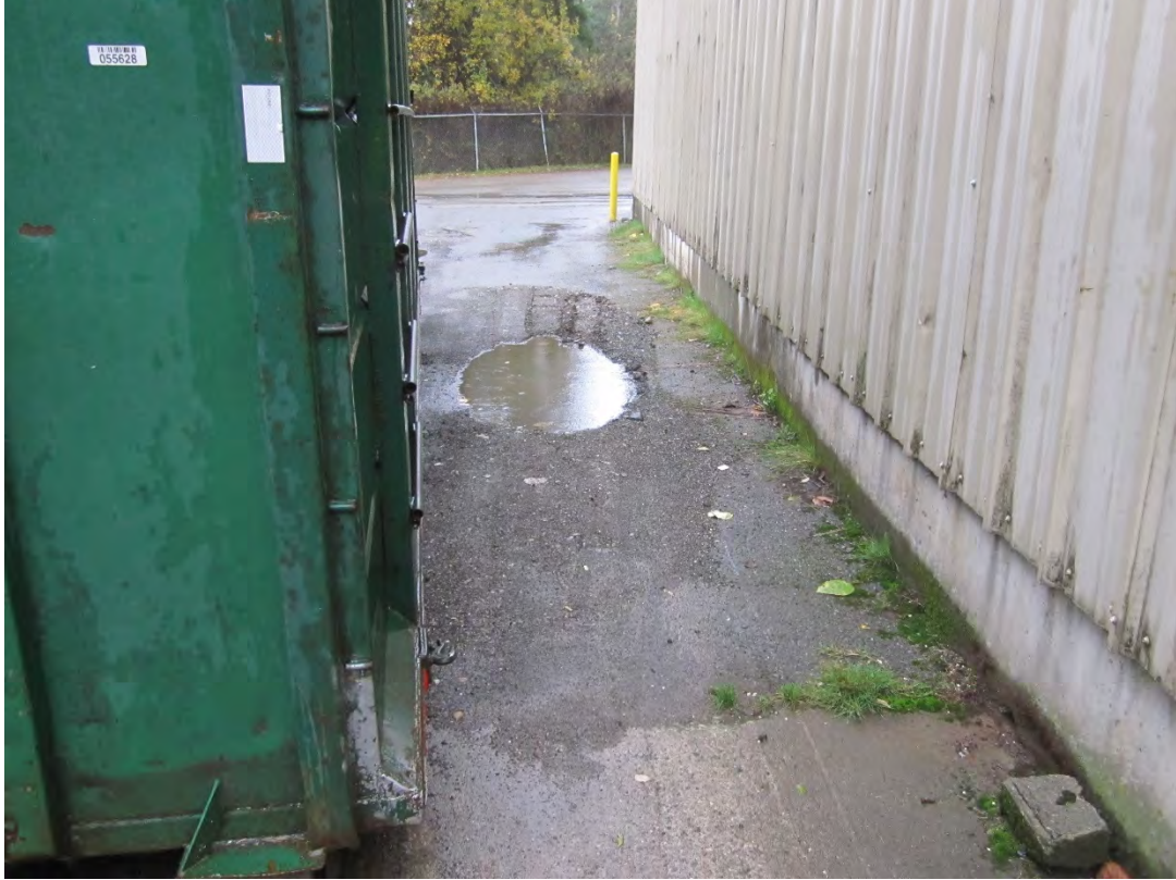
Figure 1: Pavement Deterioration East to Refuse Shed B
