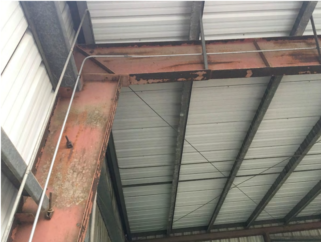
Figure 6: Shop Primer Coating Failure
