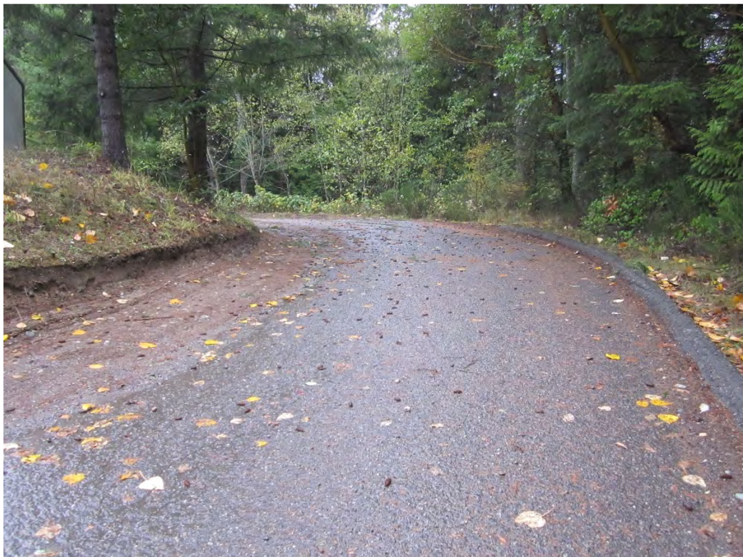
Figure 2: Rutting and Erosion on the Interior of the Haul Roadway
