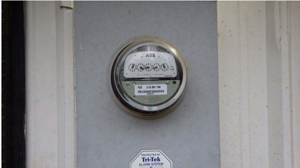
Figure 1: Electrical Service Meter
