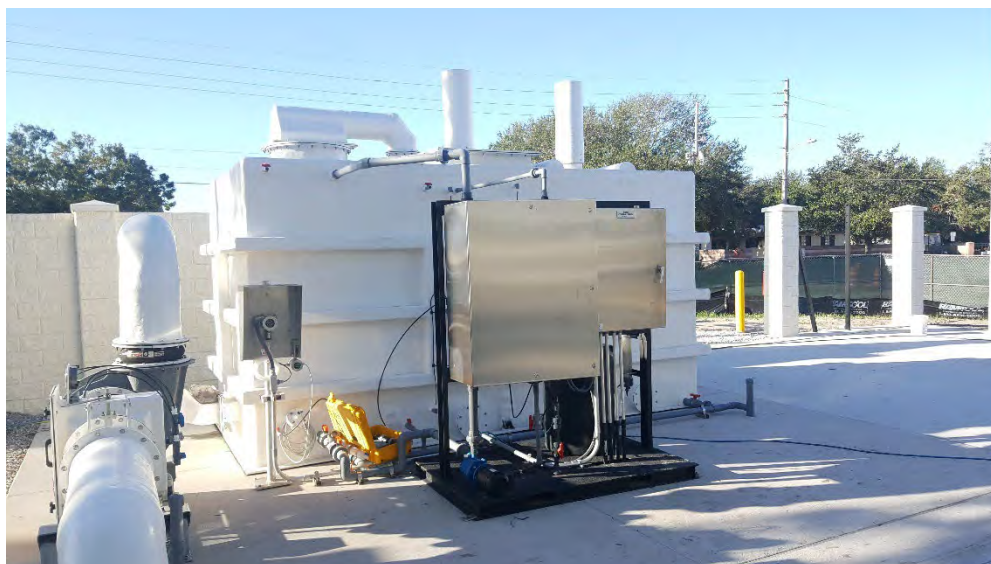
Figure 8-7 | OC-3 Engineered Biofilter
